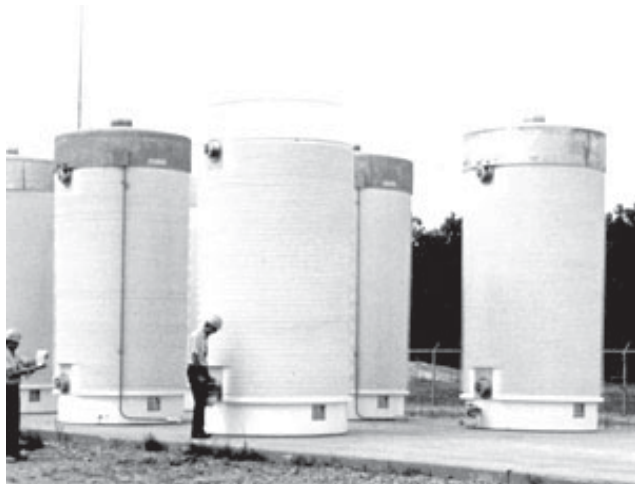
These dry storage casks are located at Xcel Energy’s Prairie Island reactor site which sits along side the Mississippi River. The Minnesota Legislature has allowed Xcel to place 48 of these containers on a concrete pad at PI. In August of 2006, Xcel petitioned for 30 dry casks at its Monticello reactor which has applied for a 20-year operating license extension.
